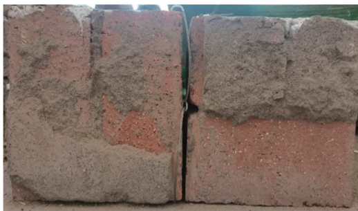
图3 破坏截面 Fig.3 Destruction of the cross-section
