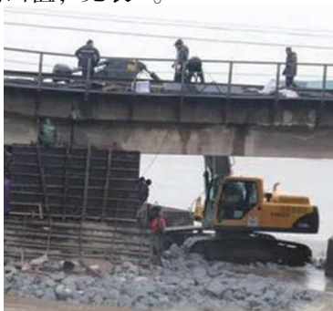
图4 实验桥梁的冲刷现状 Fig.4 Current status of experimental bridge
